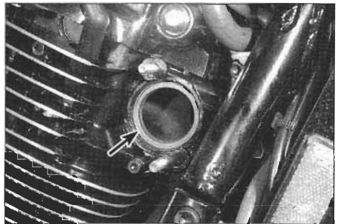
15.1c After detaching the exhaust pipes from the heads, carefully pry out the old gaskets (arrow)
